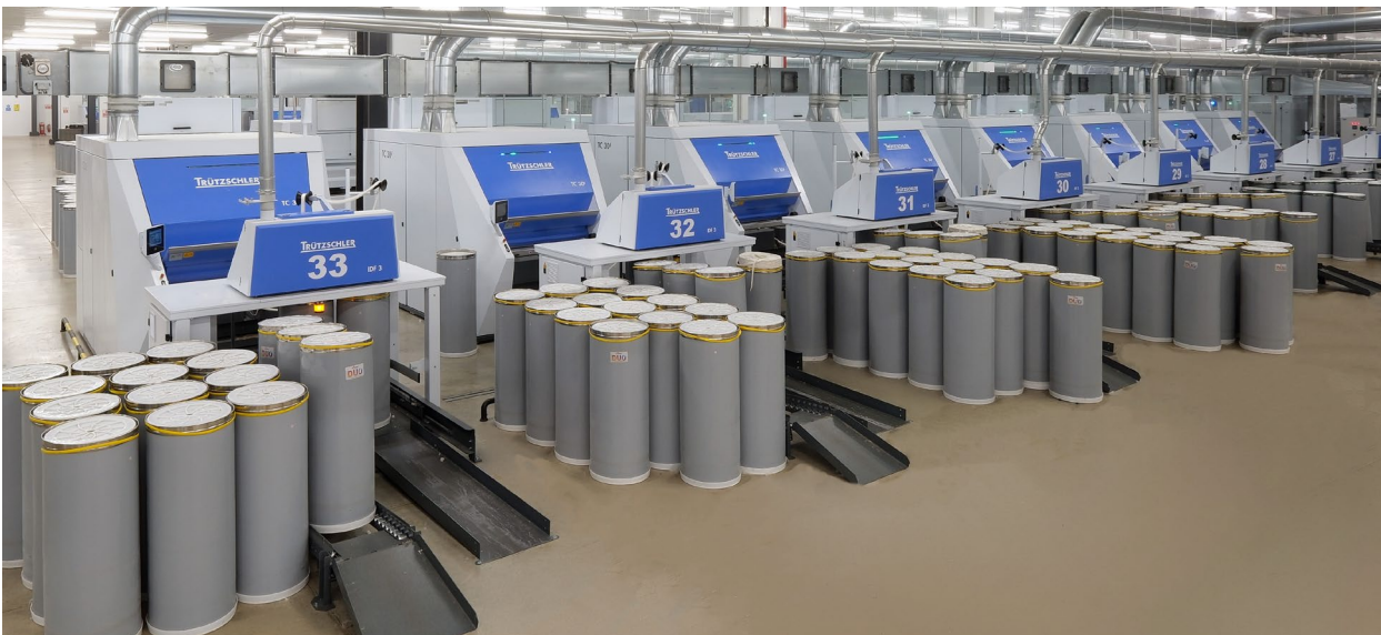
TC 30i and IDF 3 installation at a customer site in Türkiye.
